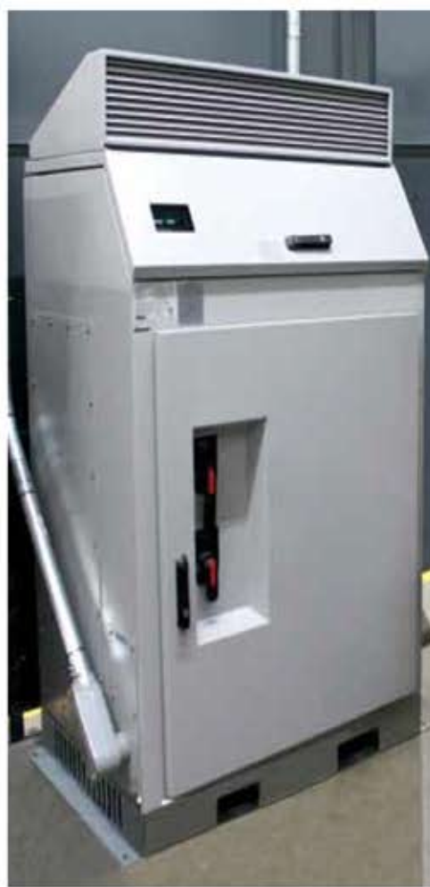
solar power inverter at ebm-papst Inc. uses ebm-papst fans
